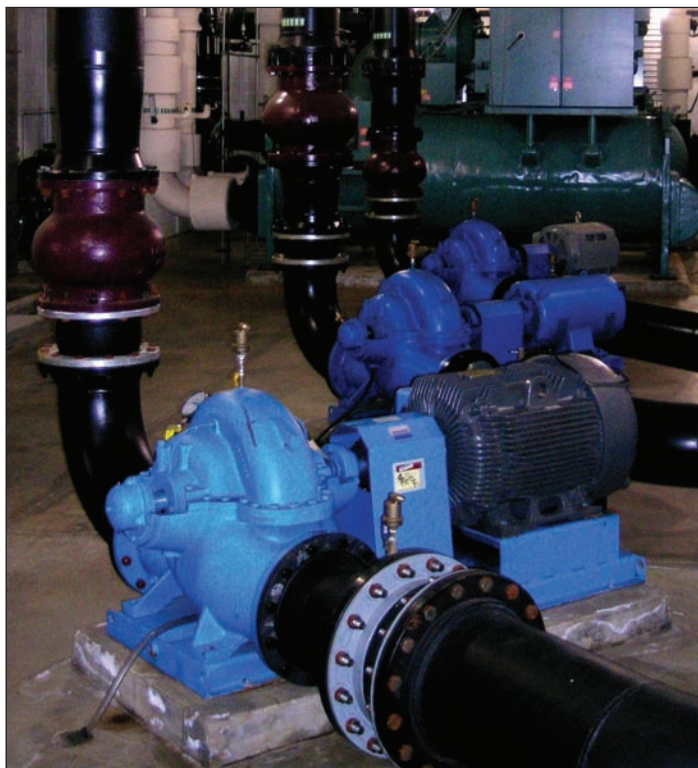
Furman University HVAC
