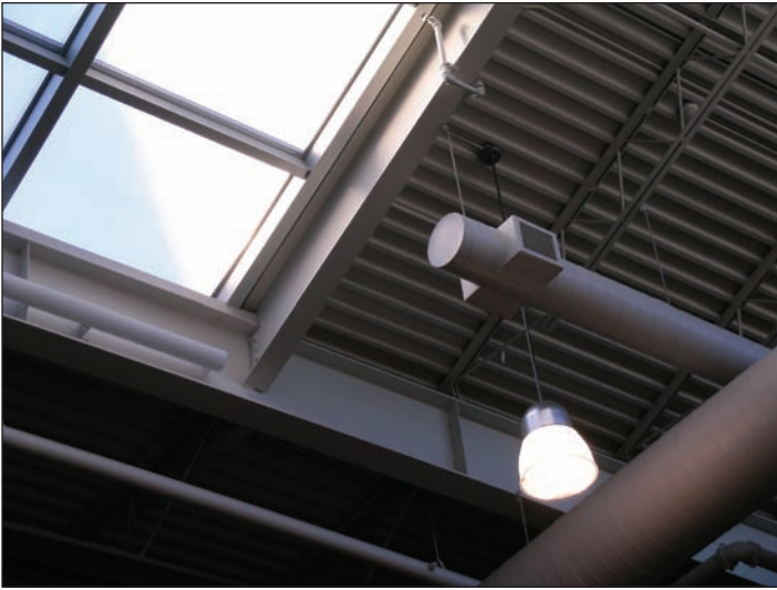
New LEED building with lights on despite full daylight
