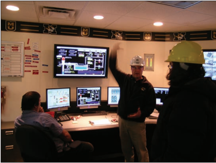
Gregg Coffin, University of Missouri’s power plant manager in the plant’s control room.
