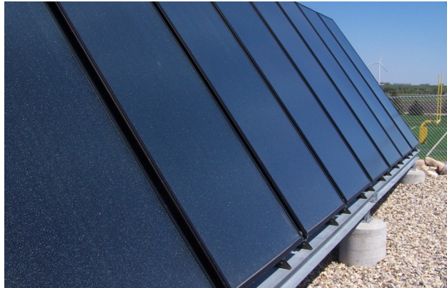
Type of System: Solar Thermal
