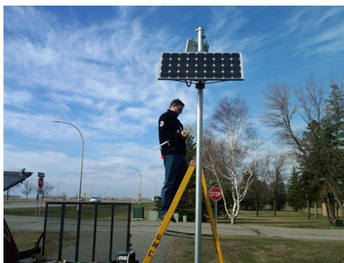
Installing the RFID bicycle monitoring unit along the UMC and community bike path.
